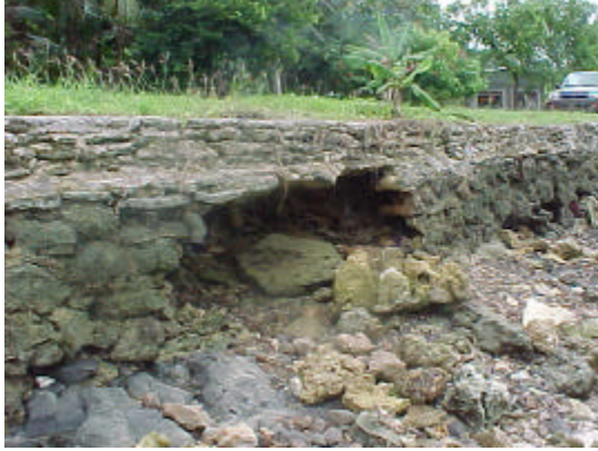
Figure 13 Damaged sea wall on Lelu Island
